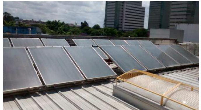
Figure 1. Solar Water Heating System and Skylights
