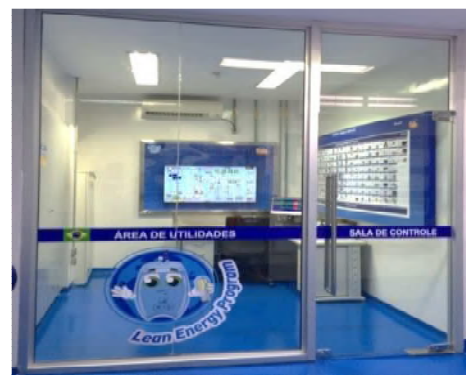
Figure 9. Utilities Control Room and Lean Energy Program Mascot Welcoming Visitors
