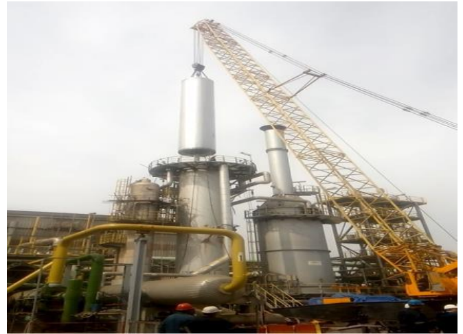
Figure 1. Ammonia Converter Basket Revamp
