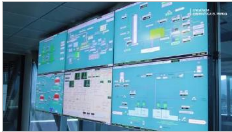
Mapocho-Trebal Biofactory's SCADA View
