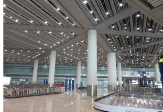
Figure 6 T3 lighting system
