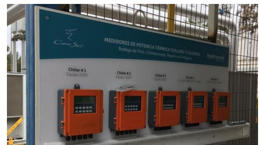
Figure 4: Wine cellar energy platform.
