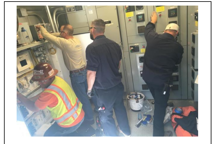
A multidisciplinary team works to improve building operations and efficiency at Berkeley Lab.
