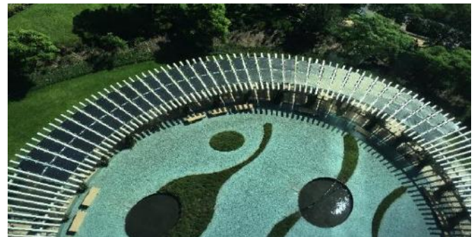
Figure 4 - Photovoltaic panels at the entrance of TPM
