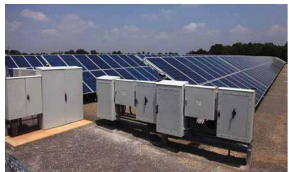
Figure 5 – Smyrna, TN Plant Solar Field – an ISO50001 certified and SEP Platinum facility
