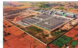
Pakistan Matri-Lahore ±660 kV HVDC Transmission Project
