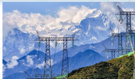
UHV/EHV Grid in Sichuan-Chongqing Region of China
