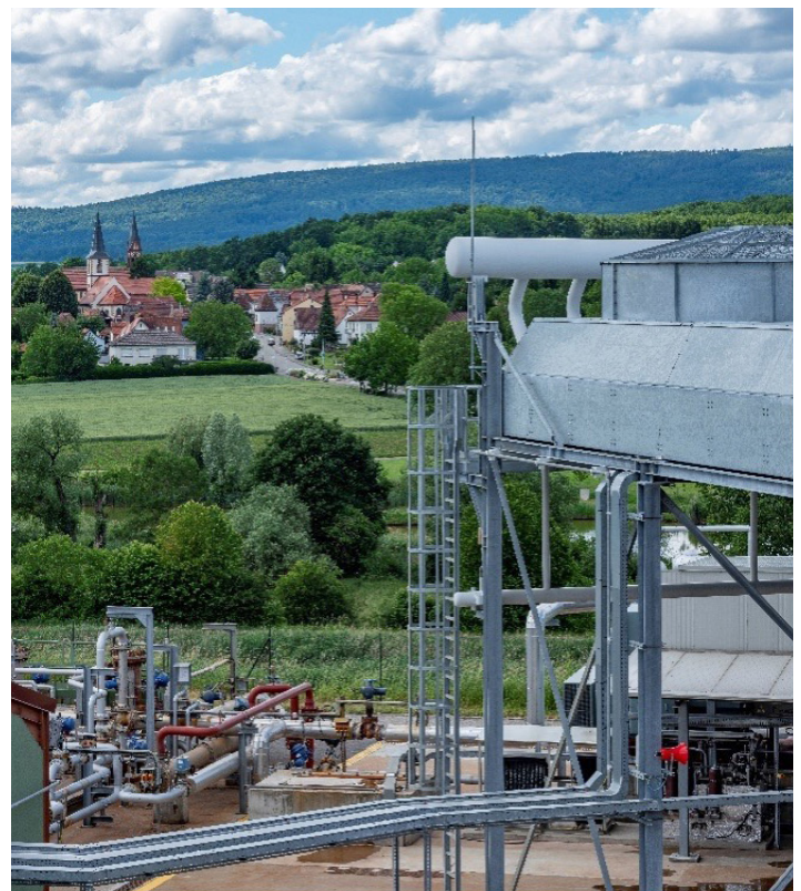
Geothermal power plant of Soultz-sous-Forêts, in the background Alsace town. Source: ES
