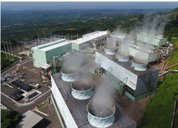
Surface facilities at the Berlin Geothermal Power Station, illustrating the heat exchange and steam separation infrastructure. Source: LaGeo
