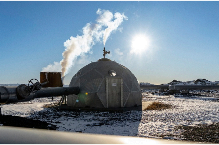
Wellhead and steam gathering infrastructure at the Hellisheiði Geothermal Power Station. Source: ON Power
