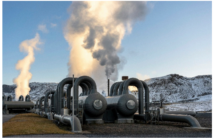
Surface facilities at the Hellisheiði Geothermal Power Station, illustrating the heat exchange and steam separation infrastructure. Source: ON Power
