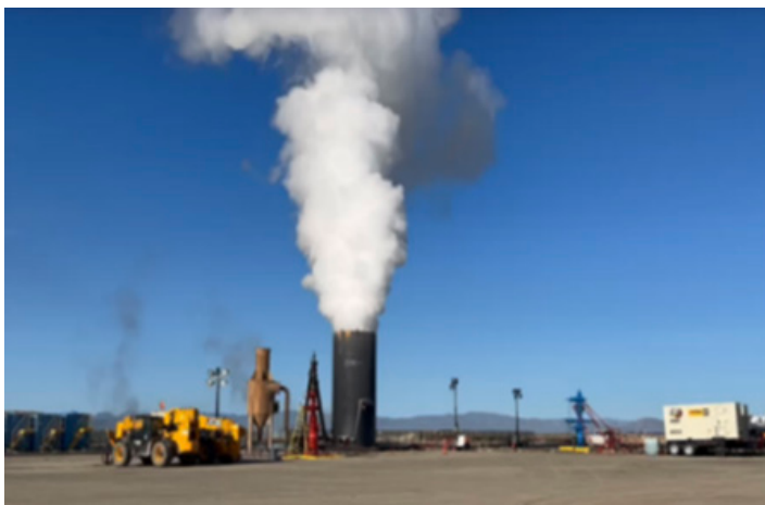
Geothermal steam testing at a Cape Station facility. Source: www.capestation.com
