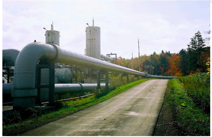
Sumikawa geothermal power station pipeline and cooling towers. Source: Mitsubishi Materials Corporation
