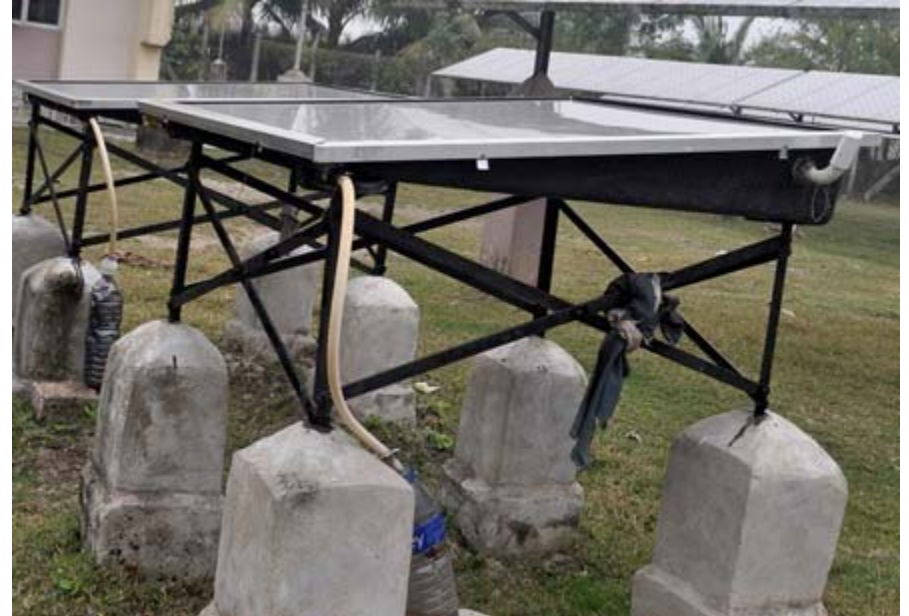
On-site distillation tables at WBREDA PV microgrid
